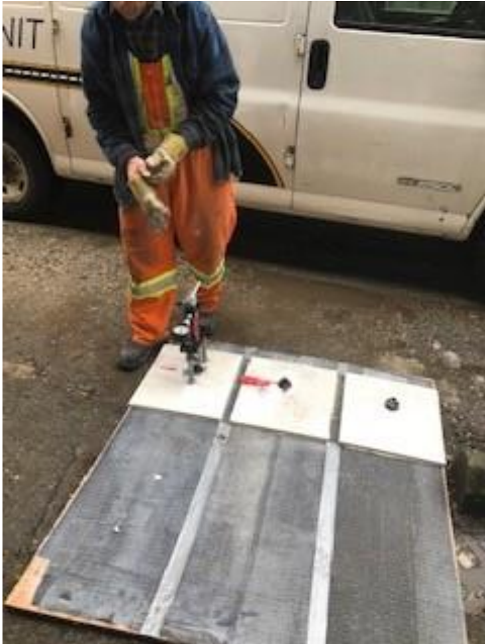
strength testing the plaster on various types of carbon wrapping to ensure the plaster will not debond
