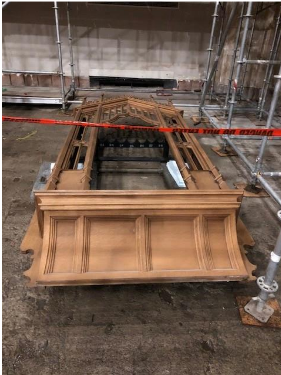
organ pipe facade taken out of the wall and places on floor
