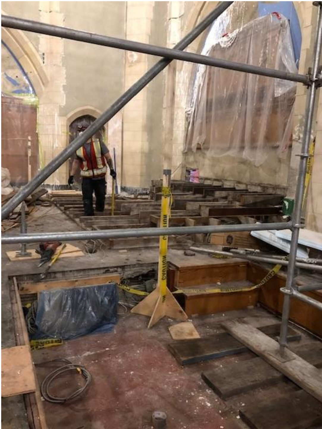
the choir pews in the chancel removed and now the platform they sit on being removed
