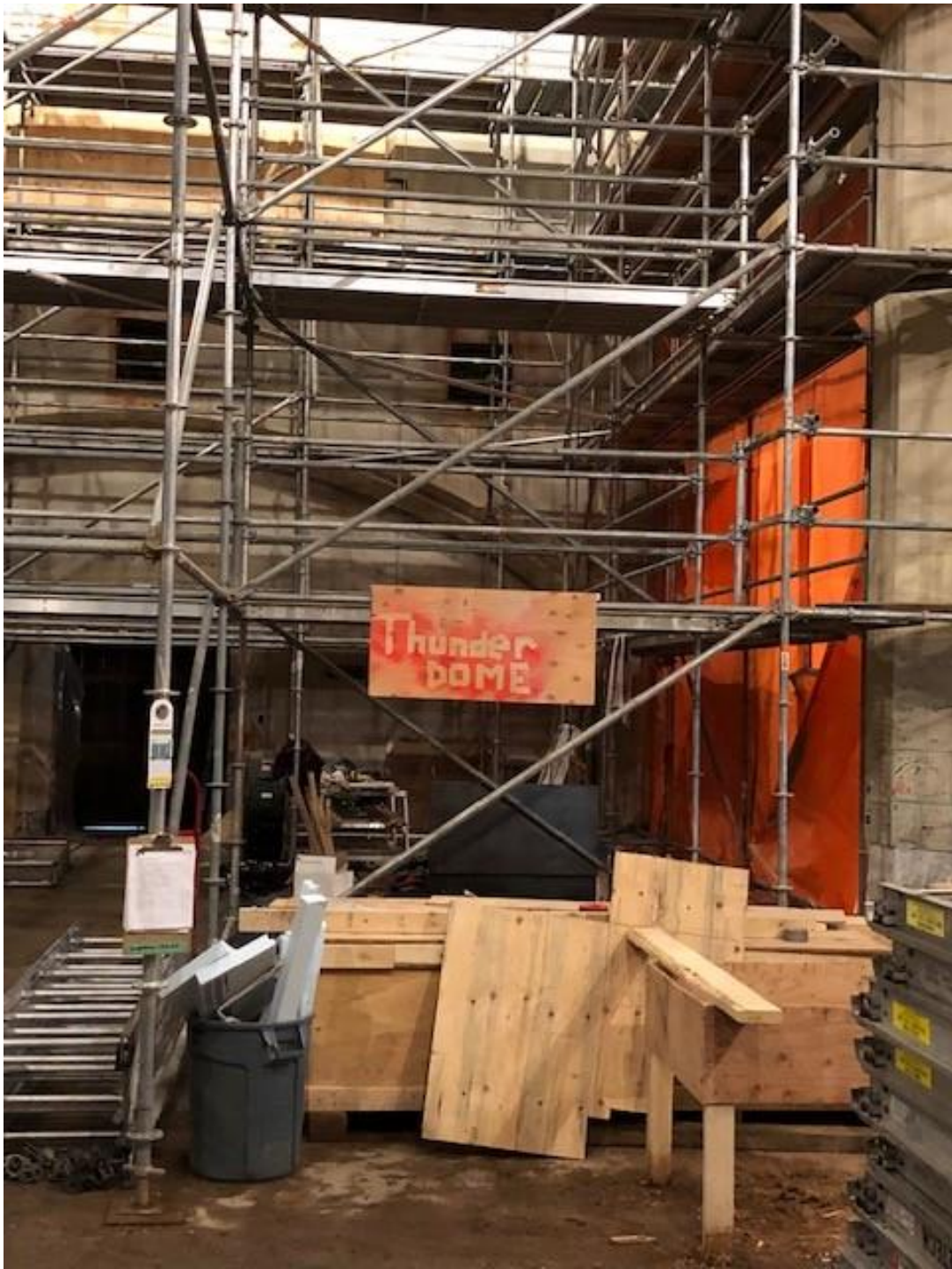
the construction workers have seen the movie MadMax and the scaffolding reminds them of a scene in the film
